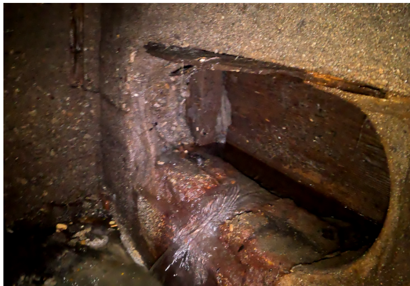
tide leaking through tide gate into inlet chamber
