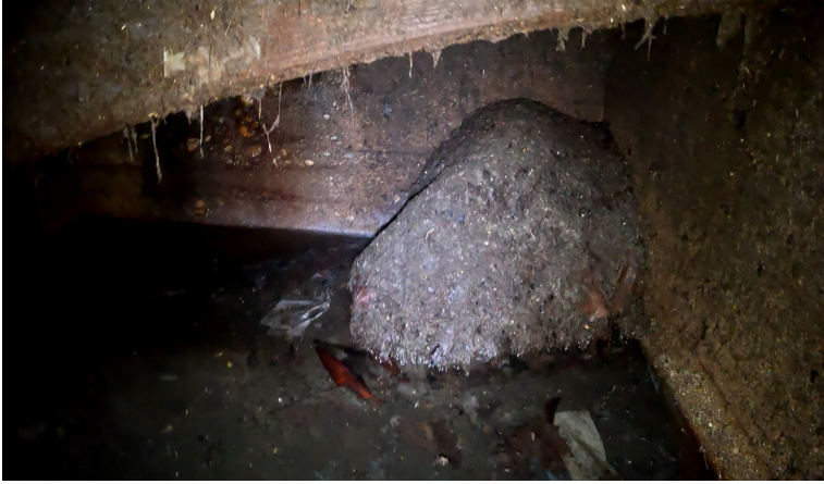
big lump in tide chamber- maybe covering outlet?
