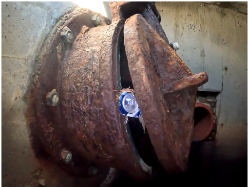
propped open flow gate
